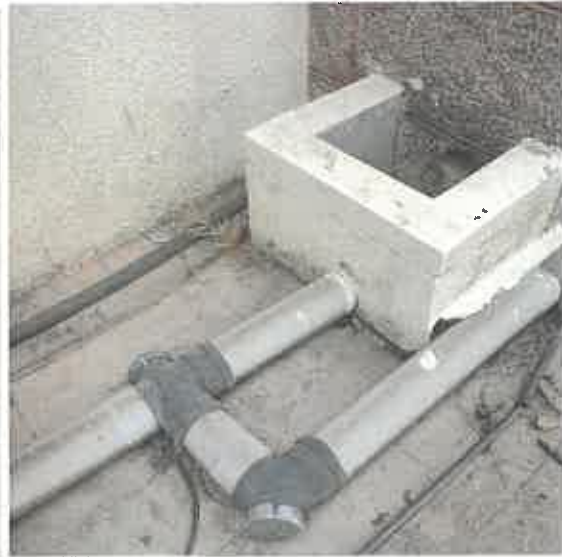
Pipeline for Rainwater Harvesting
