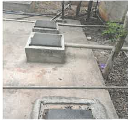
Domestic Water Sump – 2 lakhs litre capacity
