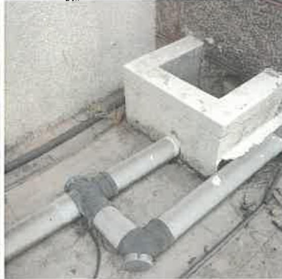
Pipeline for Rainwater Harvesting
