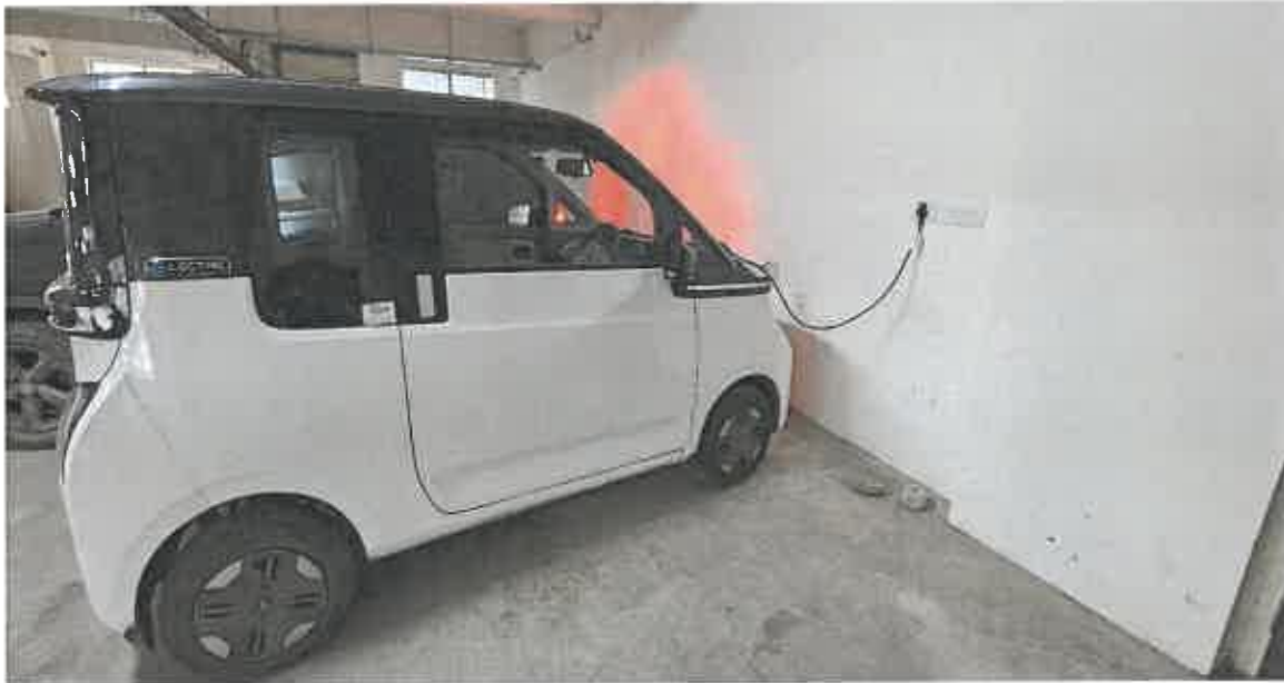
Charging points for E vehicles
