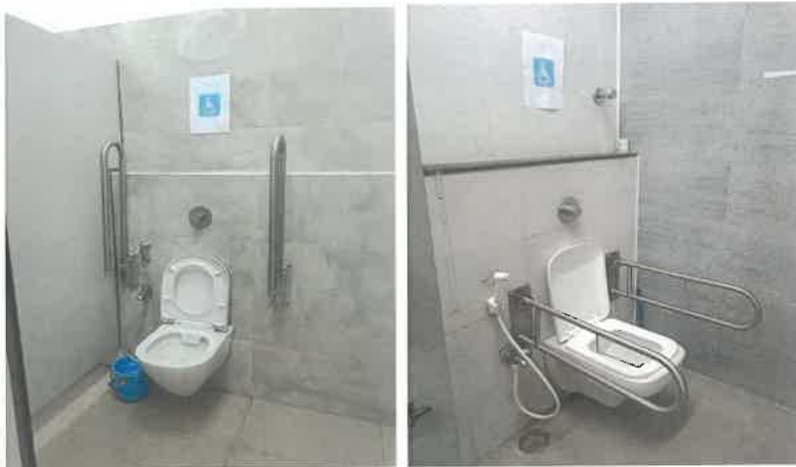
Washroom facility for differently abled
