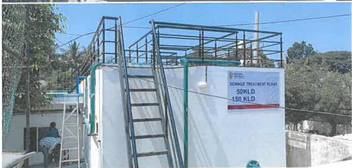
STP 50 & 150 Tank at RT Campus
