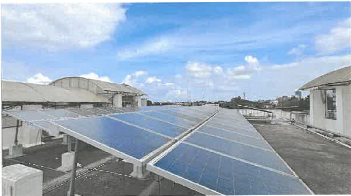
Solar panels on roof top
