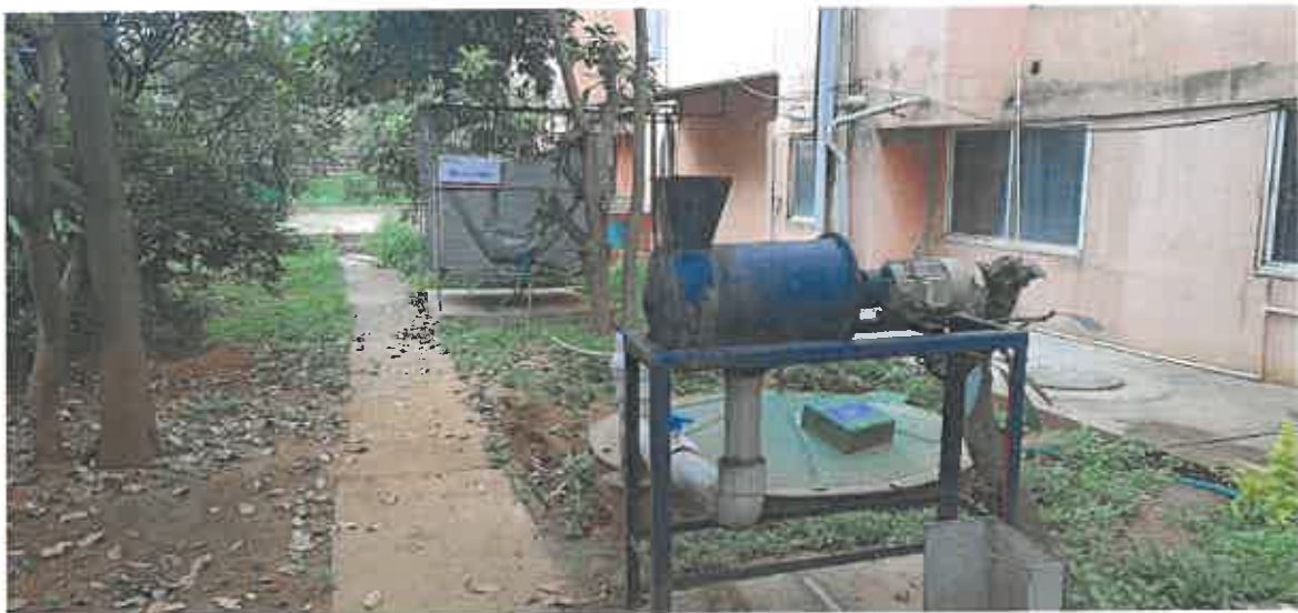
Biogas plant at RT campus
