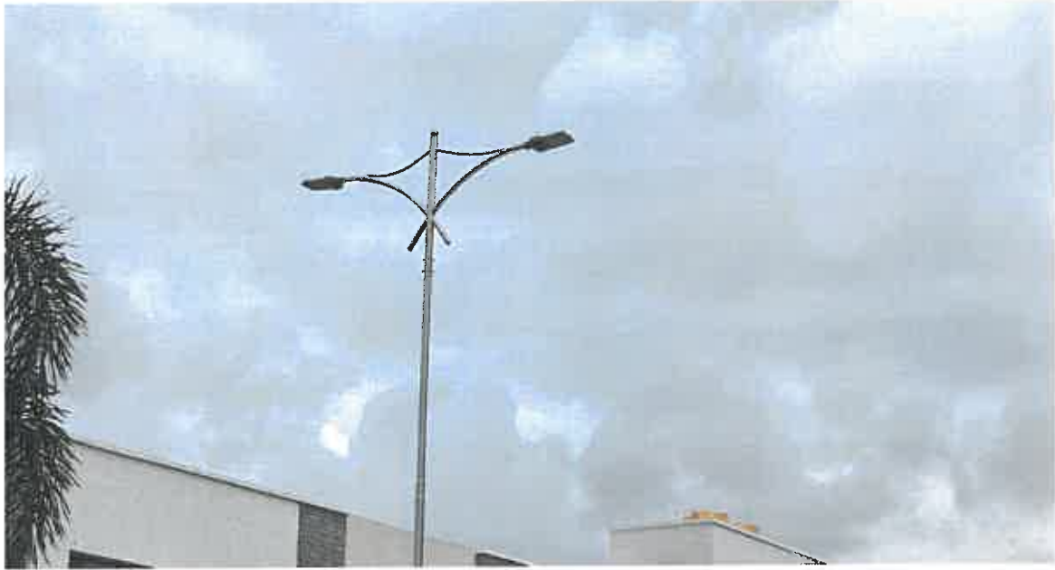
LED Lighting Distribution for Outdoor Street Area Light
