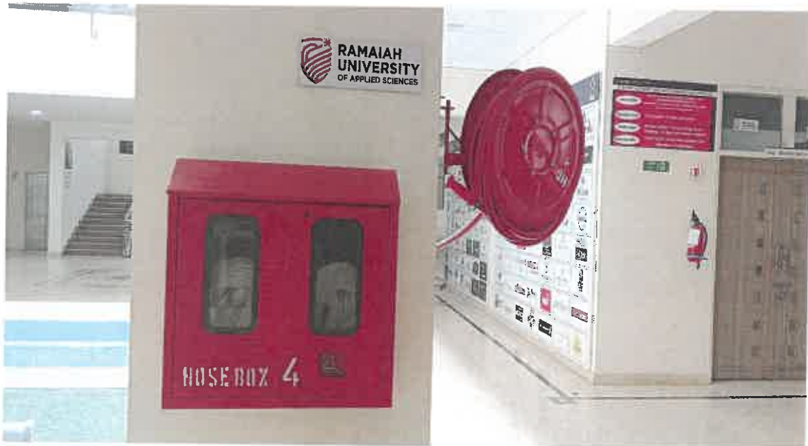
Fire suppression system
