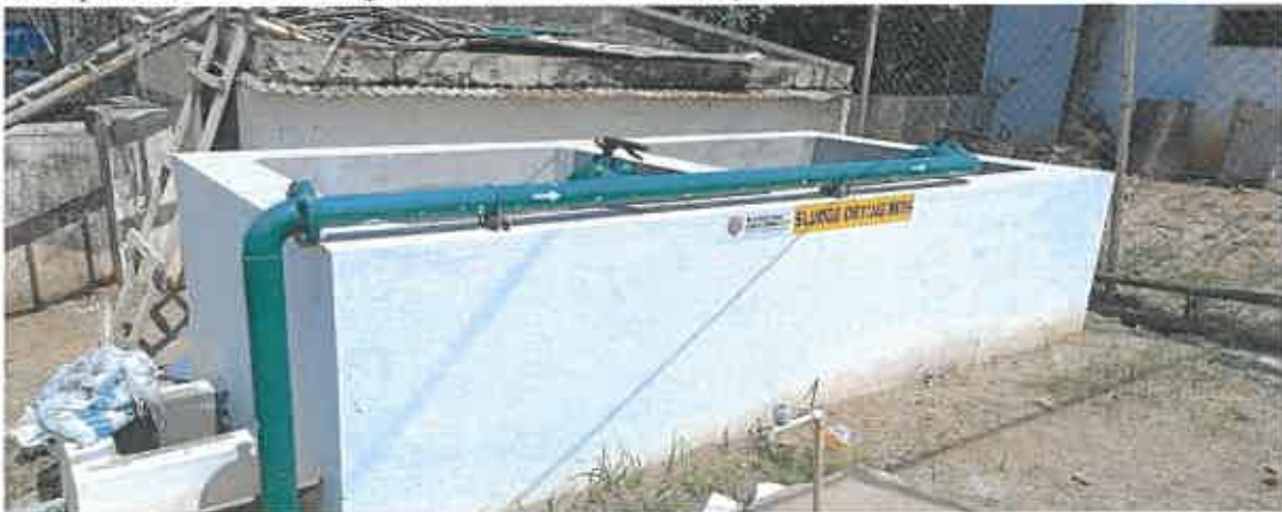
STP 50 & 150 Tank at RT Campus
