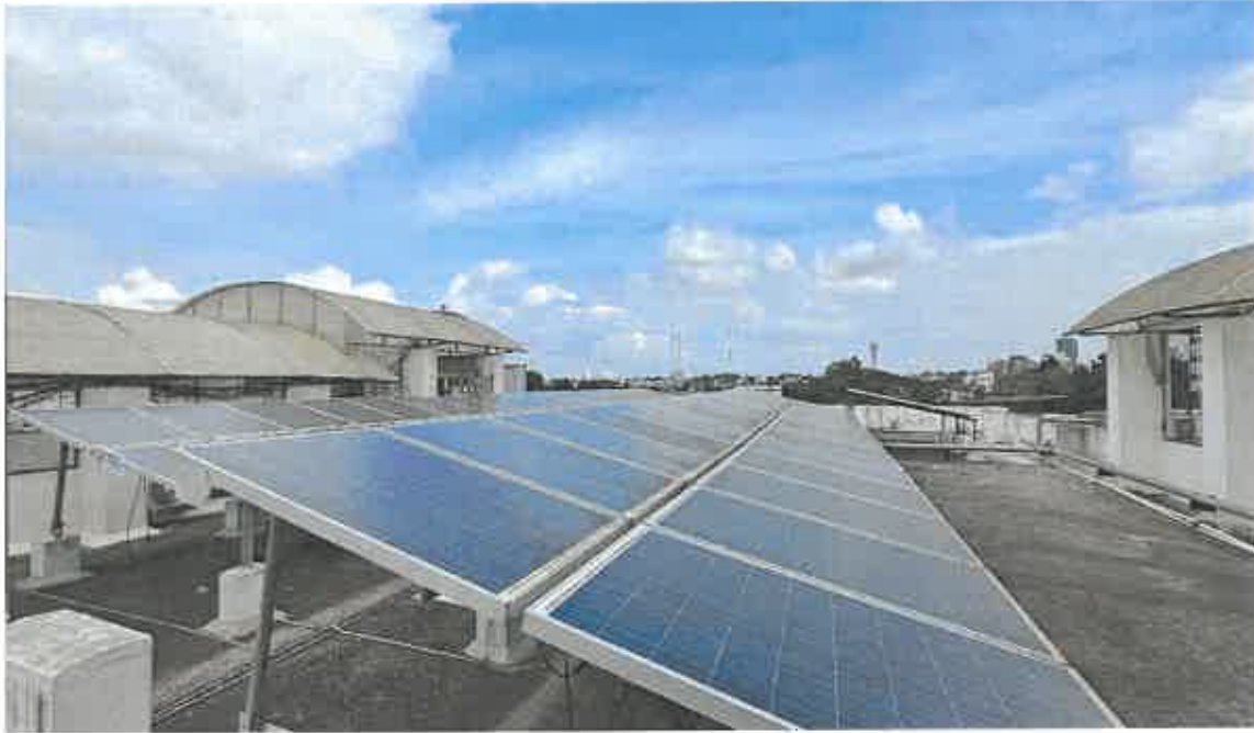
Solar panels on roof top
