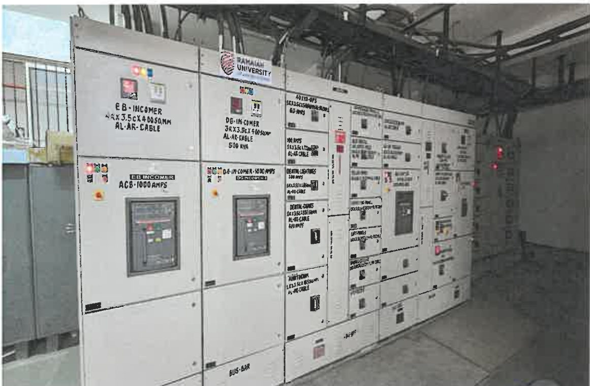
Control panel room at Gnanagangothri Campus
