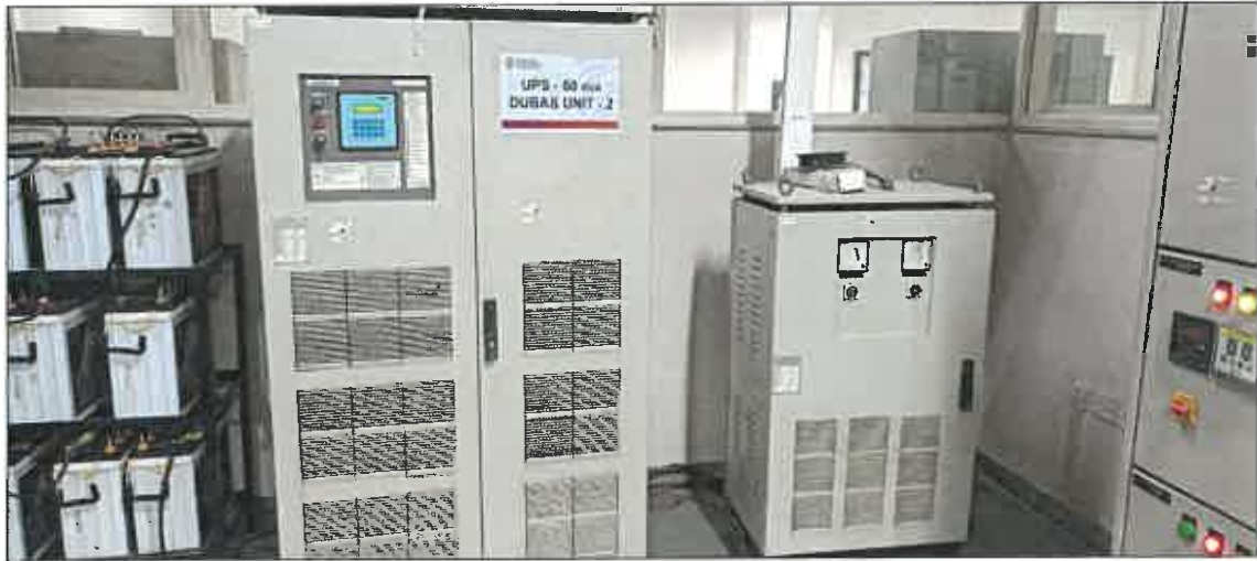
60 KVA Dubas UPS with Isolation Transformer (B Block)
