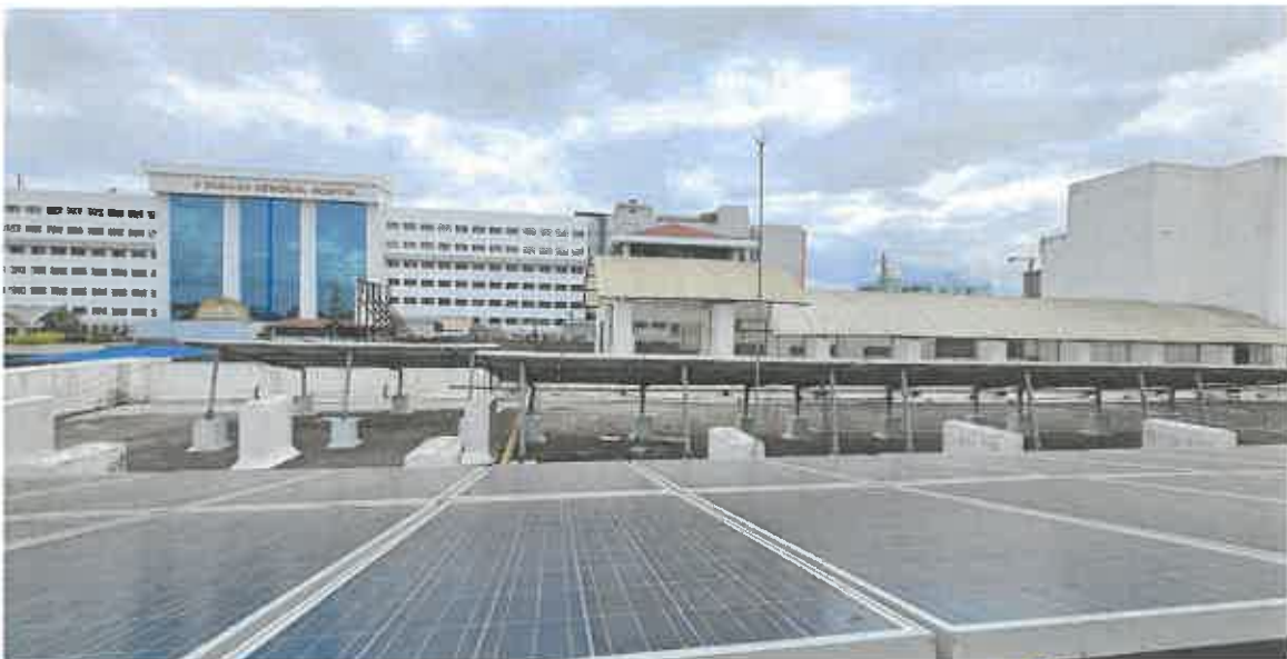
20 KWp Solar System
