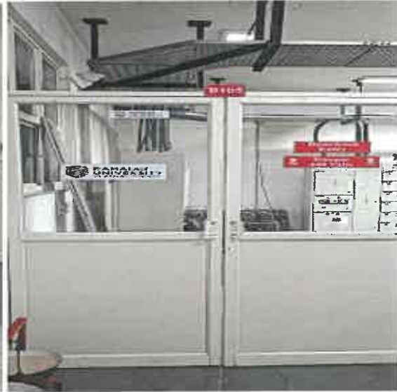
UPS Room (B Block)
