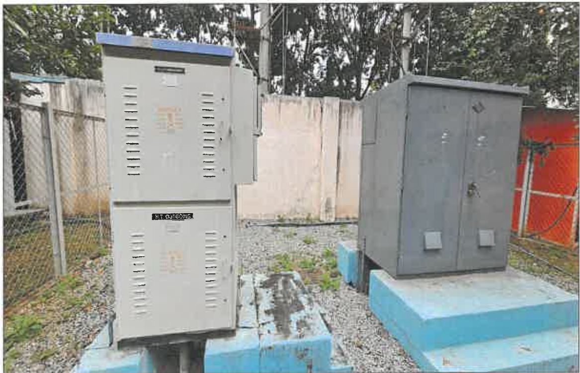
Sub station at RT Campus
