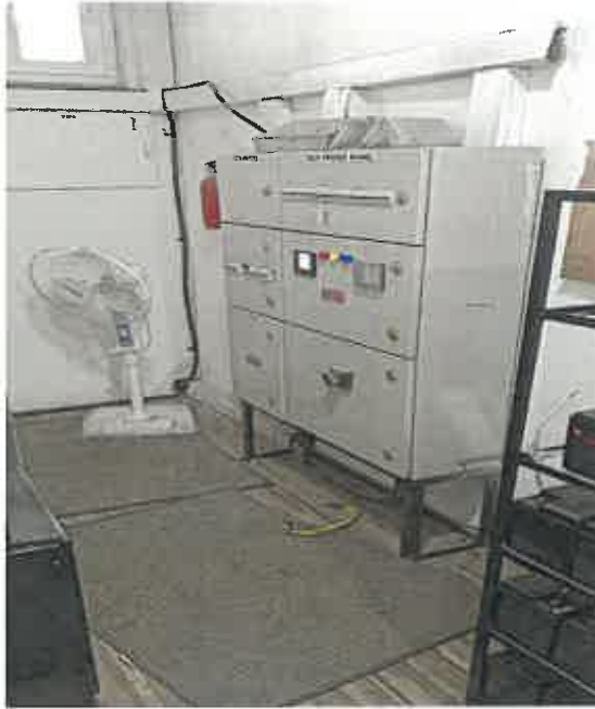
Techno Block UPS Room & Control Panel
