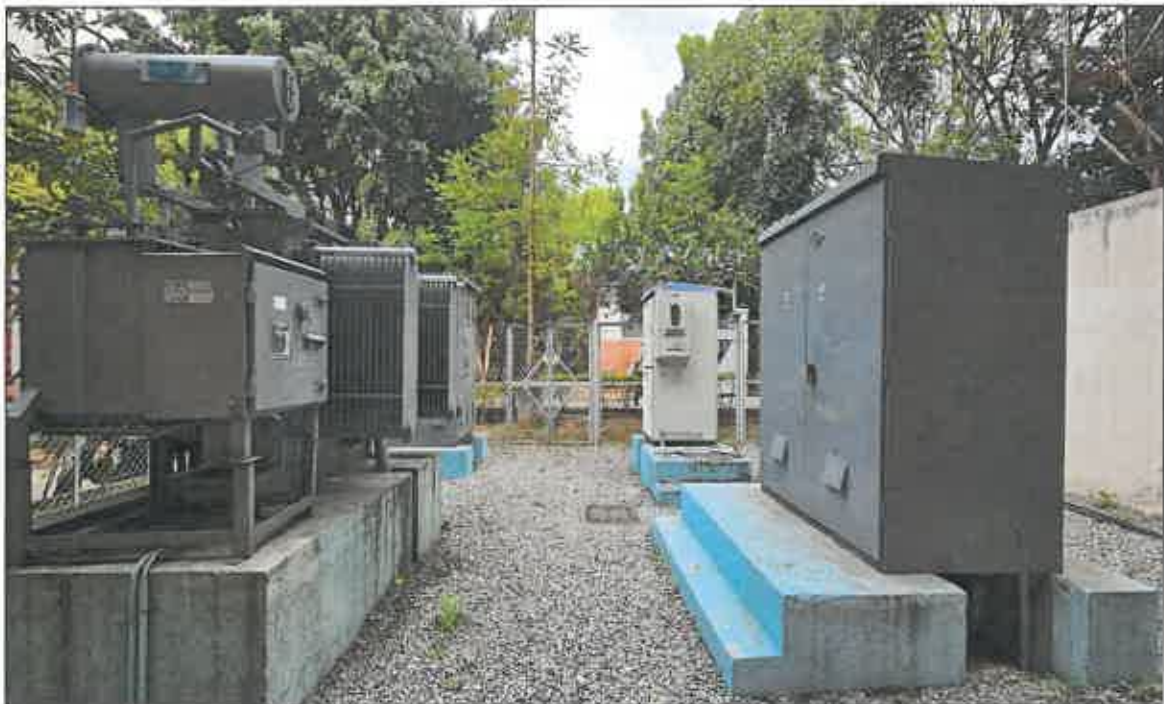
Transformer at RT Campus
