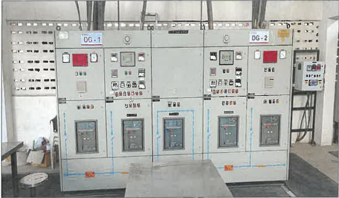
DG Control Panel
