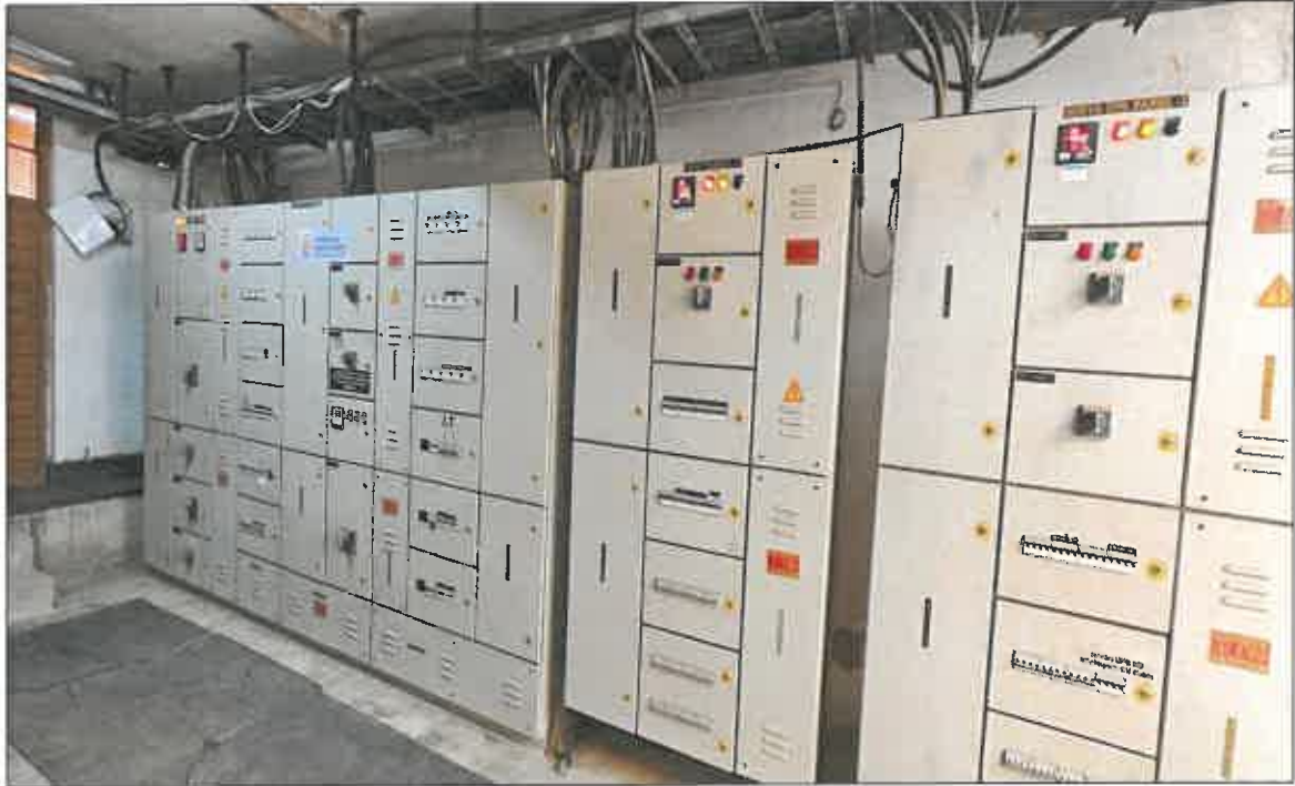
Control panel room at RT campus
