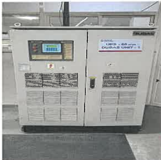
60 KVA Dubas UPS (B Block)
