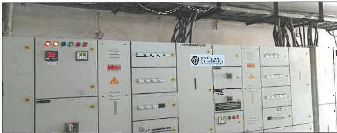
C & D Block Control Panel
