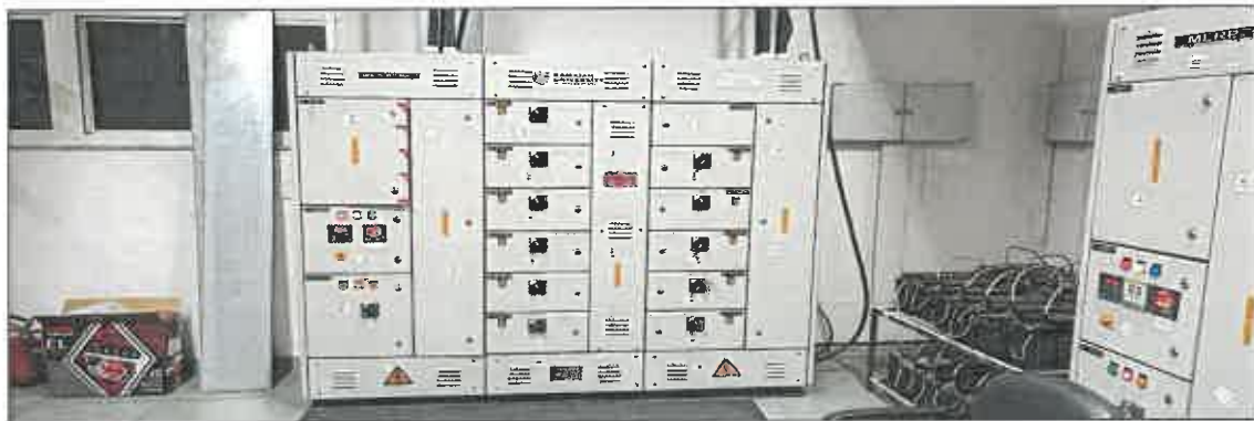
UPS Power Panel
