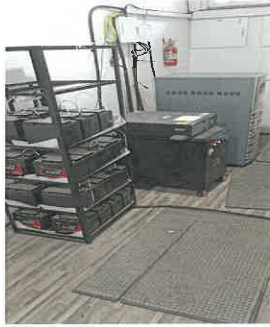
20 KVA UPS (Techno Centre Block)
