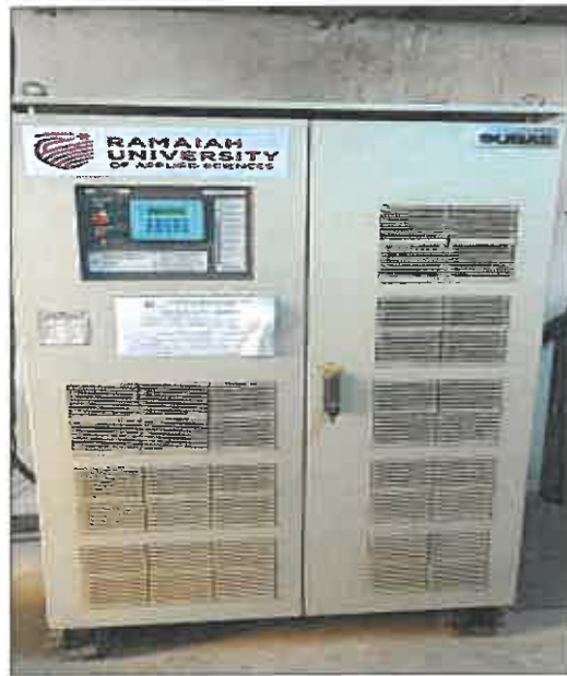
C & D Block 80 KVA Dubas UPS
