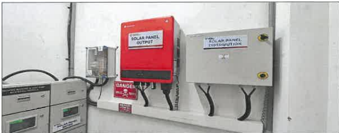
Solar Plant 35KWp and solar System
