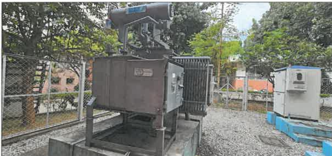
Transformer at RT Campus
