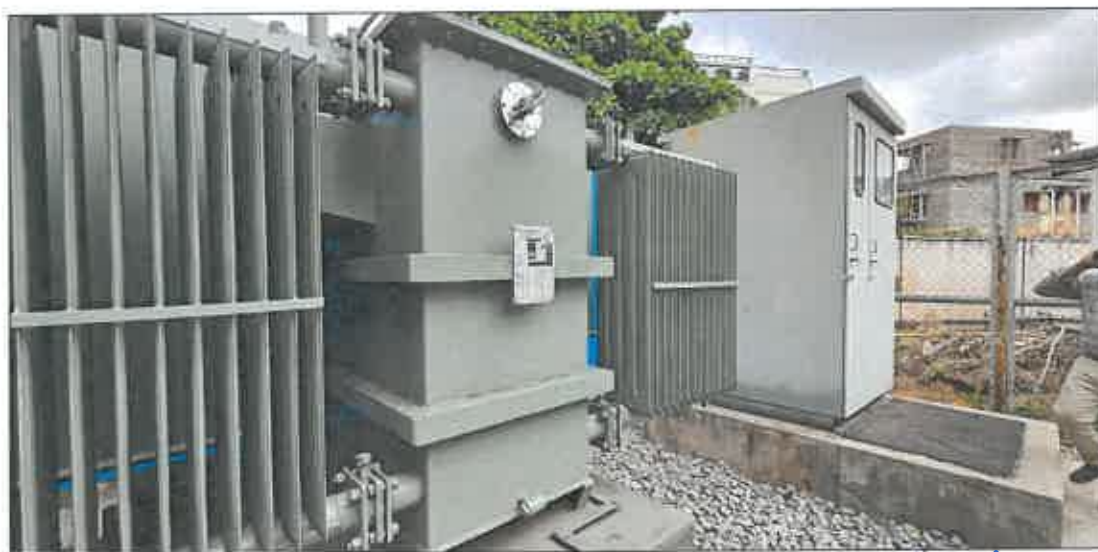
Figure: - 1000 KVA Transformer
